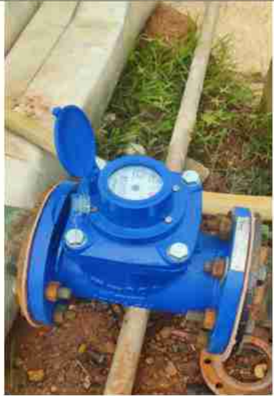
Photograph of water flow meter
