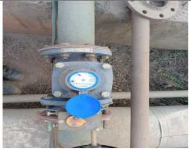
Photograph of water flow meter
